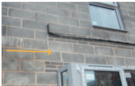
The greater the distance between lintel level and roof intersection DPC/tray level, the greater the susceptibility to damp permeating horizontally across the bay.
