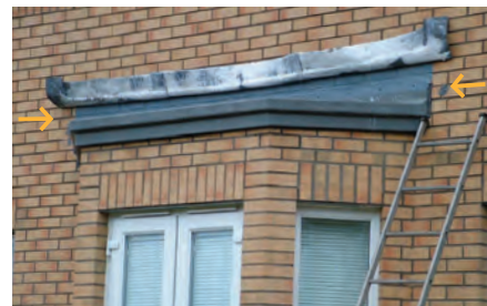
The extensive fascia height means there are a considerable number of masonry courses between the bay support lintel and the higher roof/tray intersection level. To prevent damp permeating between the two it is necessary to incorporate a vertical link whilst maintaining coursing and bond.
